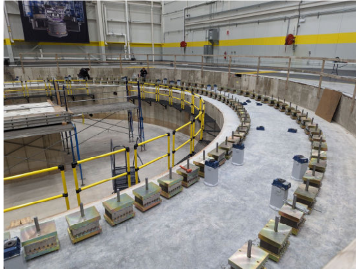
Figure 13. The GMT Mount “test pit” area in the high bay facility at IMT in Rockford, IL. For factory integration and testing, this area represents the top of the GMT pier that interfaces with the Mount’s azimuth track. The “springbox” assemblies, just one type of the multiple components and assemblies that are part of this complex interface, are shown here as they are being laid out for the azimuth track integration later this year. (Photo courtesy of Ingersoll Machine Tools)
